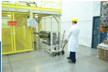
6. Push-off mechanism is retracted & the cart is manually removed from the winder stall
